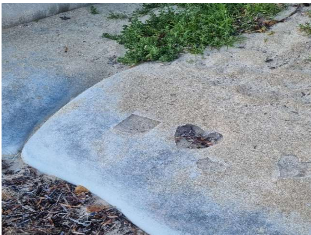
Figure 8-1: Photo taken of vandalised GSC located within the Flinders Ln seawall, approximate chainage +3300 m. Taken during site visit 18 September 2024.
