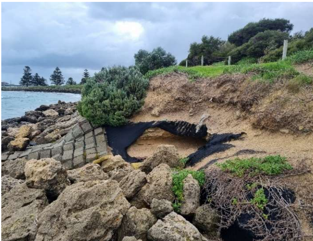
Figure 7-9: Damaged geotextile along seawall crest (+1100m), adjacent to old boat ramp, taken during site visit 14/08/2024.
