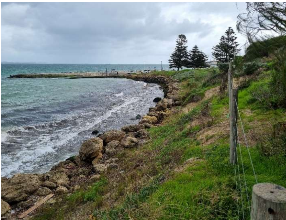
Figure 7-7: Limestone seawall (+1100m) south of Wells Park, showing eroded dune face above, facing northwest during site visit 14/08/2024.
