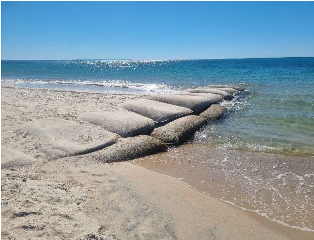
Figure 11-25: GSC Groyne 9 with damaged bag spilling sand (+1240m) taken during site visit 27 November 2024.
