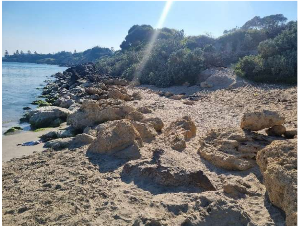
Figure 7-12: Limestone seawall south of Wells Park (+850m), showing southern end, facing east during site visit 18/09/2024.
