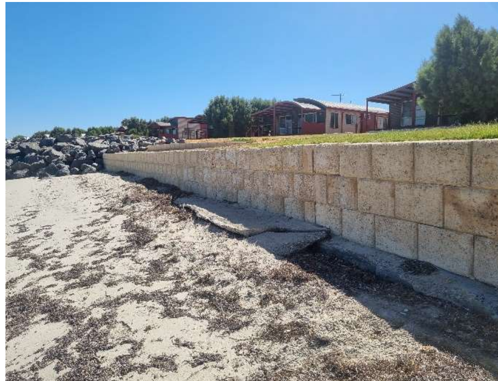
Figure 1-5: Ad hoc repairs/cracking of poured concrete supporting retaining wall at Grannies beach (taken during site visit 29 January 2024)
