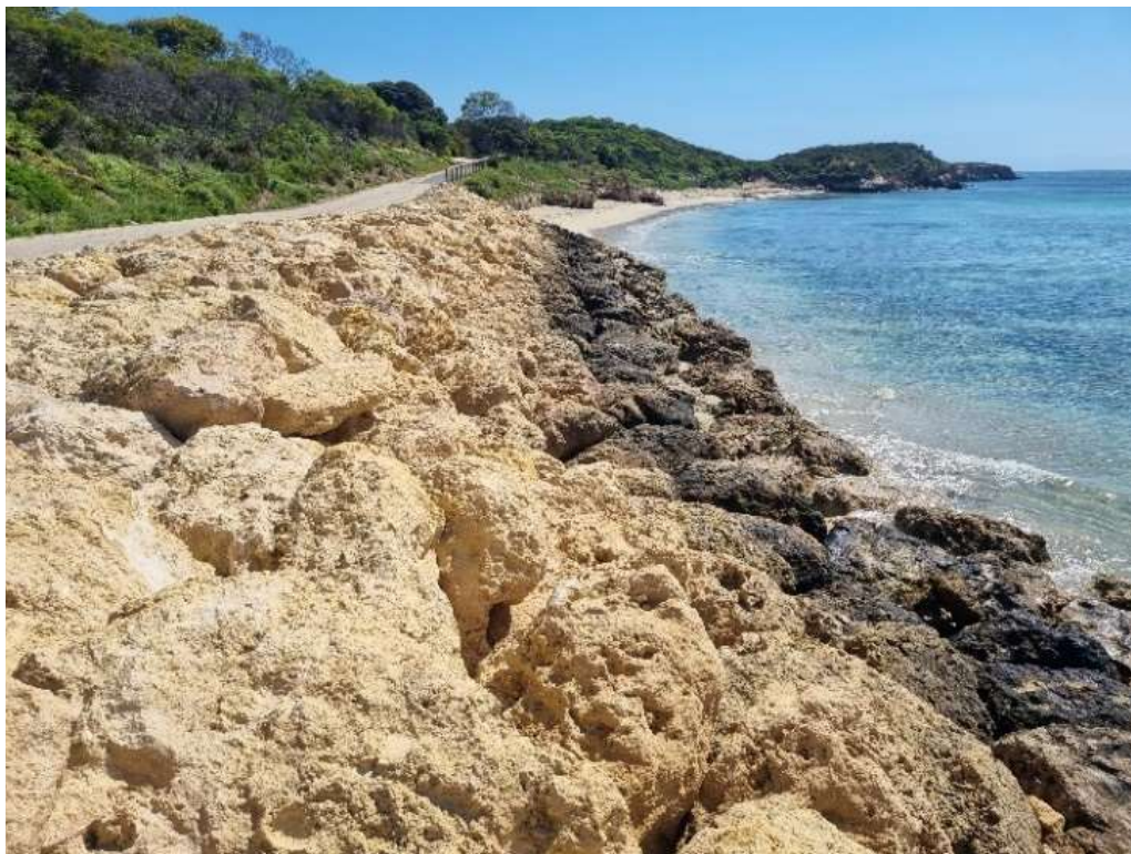
Figure 9-7: DBCA Revetment (+1200m). Taken during site visit 18 September 2024.
