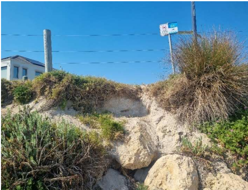
Figure 8-17: Slope erosion at Hymus St. informal seawall (+1375m). Taken during site visit 18 September 2024.
