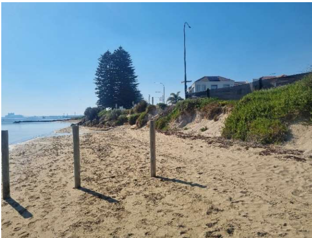
Figure 8-19: Scarping present immediately west of Hymus St. informal seawall (+1300m). Taken during site visit 18 September 2024.
