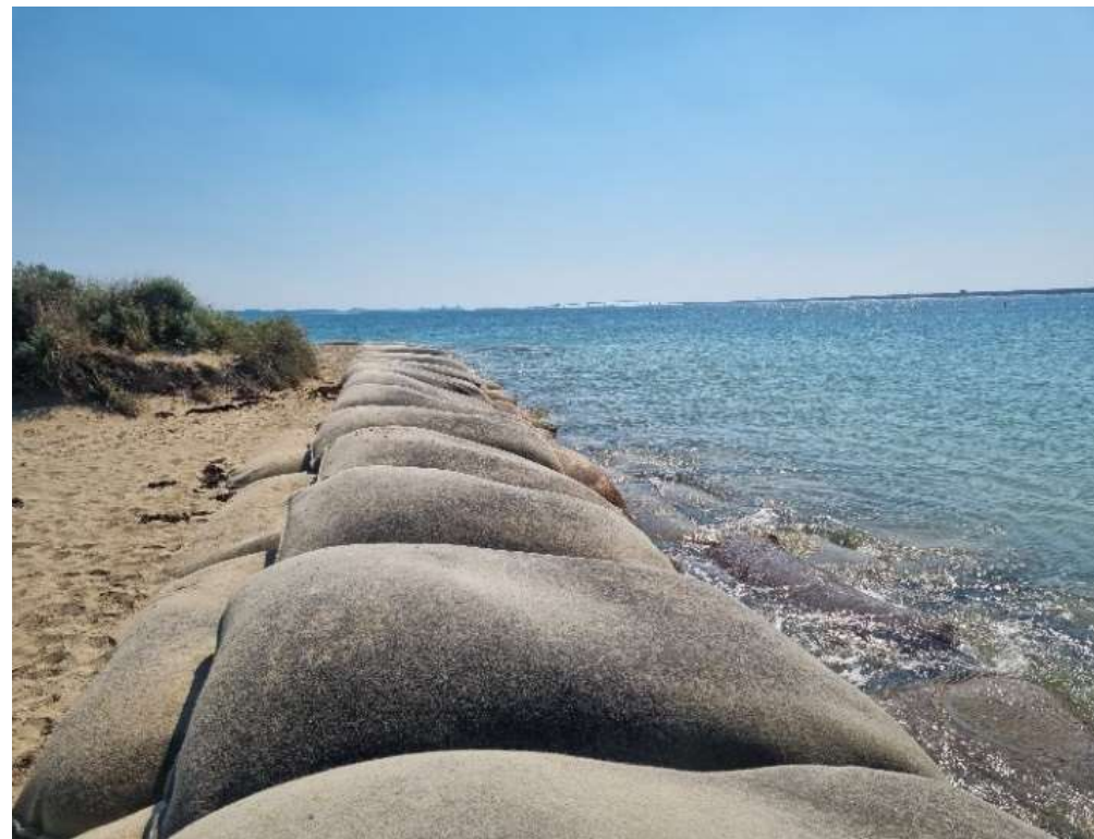
Figure 9-2: Sagging GSC groyne. Taken facing north during site visit 18 September 2024.
