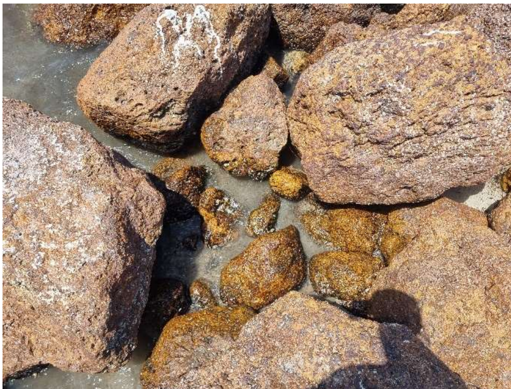
Figure 11-4: Groyne 1 (+250m), laterite rock core exposed with minimal armour cover. during site visit 27 November 2024.
