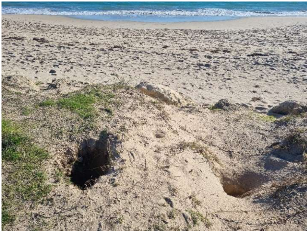
Figure 10-1: Photo taken of voids at crest of Town Beach seawall, approximate chainage +325 m. Taken during site visit 1 July 2024.
