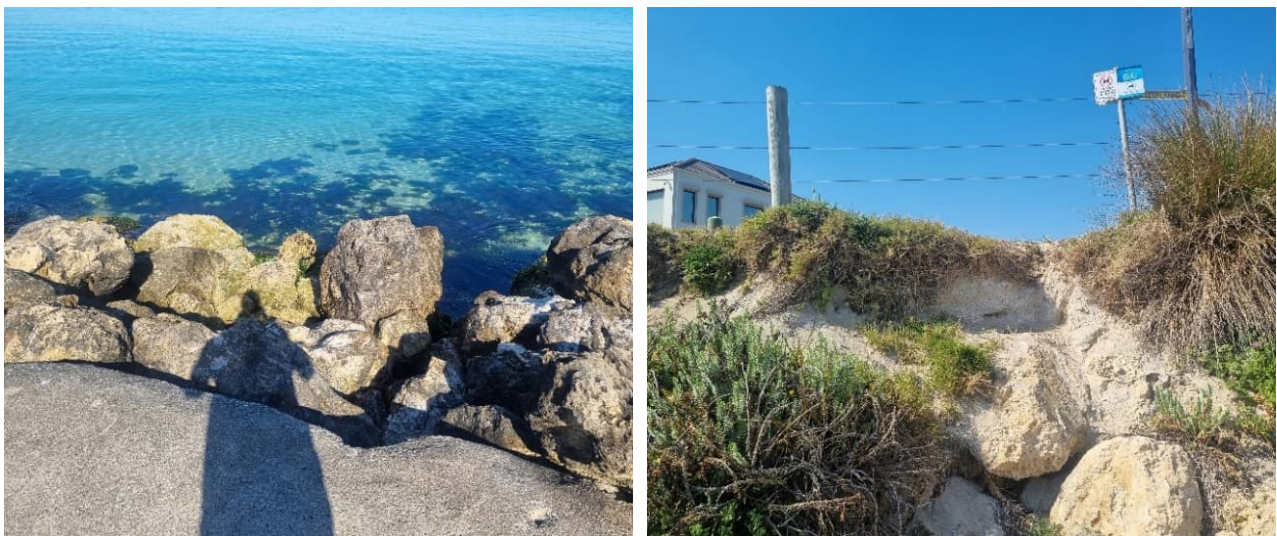
Figure 2-3: (left) Wells Park headland/revetment (Kwinana Beach) with poor interlocking of armour material (right) Informal seawall at Hymus St. (Rockingham Town Beach) with erosion from overtopping and omission of lack of filter layer and geotextile
