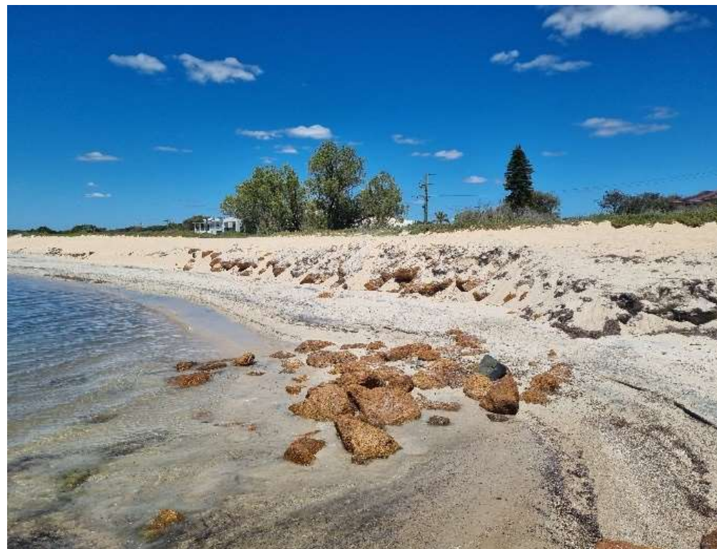
Figure 11-6: Immediately north of Groyne 2, laterite armour rock scattered on beach and informal seawall present (+360m) taken during site visit 27 November 2024.
