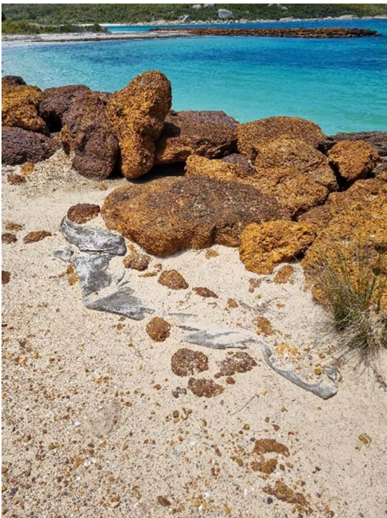
Figure 12-15: Exposed geotextile along seawall (+600m) taken during site visit 5 December 2024.
