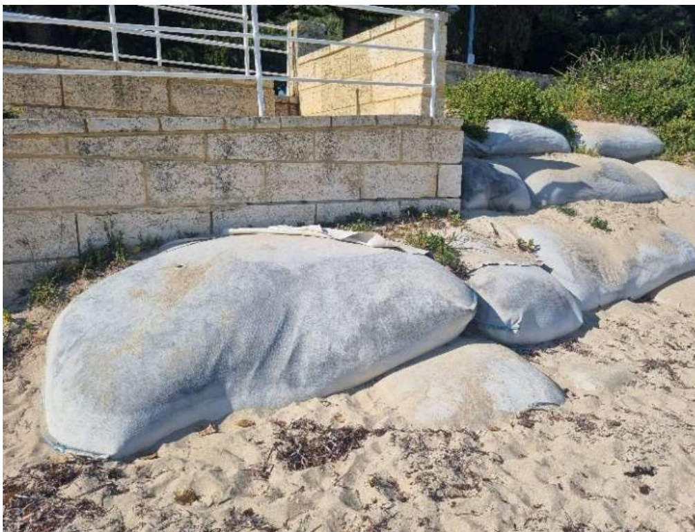
Figure 8-5: Photo taken of damaged GSC within the Flinders Ln seawall, approximate chainage +3375 m. Taken during site visit 18 September 2024.
