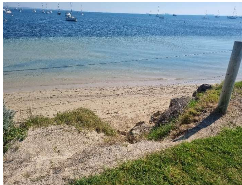
Figure 8-20: Slope erosion at Hymus St. informal seawall (+1375m). Taken during site visit 18 September 2024.
