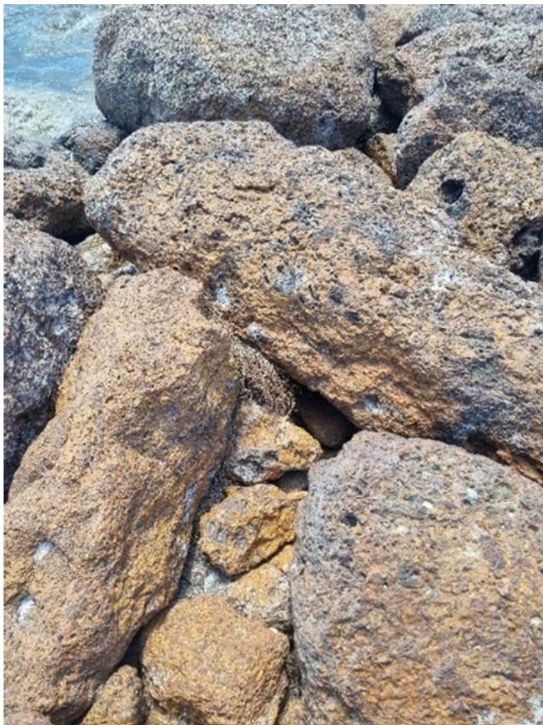
Figure 11-3: Groyne 1 (+250m), laterite rock core exposed with minimal armour cover. during site visit 27 November 2024.
