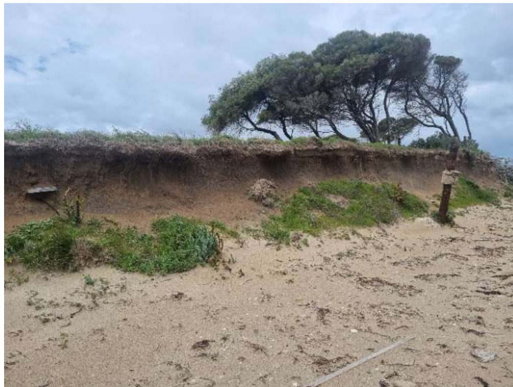
Figure 6-4: Coastal scarping and damaged ground water monitoring wells (chainage +2750m), taken during site visit 14 August 2024.
