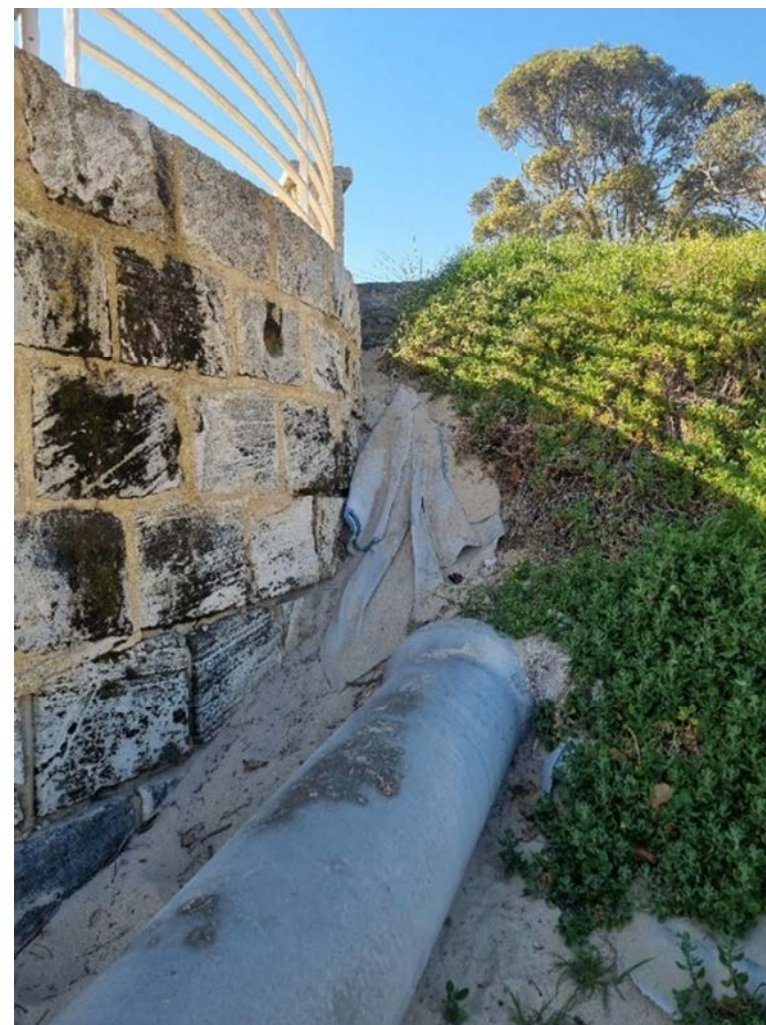
Figure 8-2: Photo taken of empty/damaged GSC within the Flinders Ln seawall, approximate chainage +3300 m. Taken during site visit 18 September 2024.
