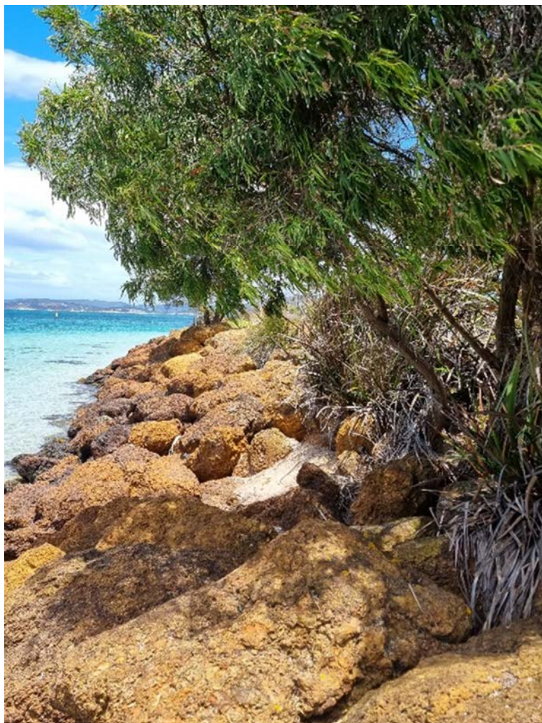
Figure 12-5: Exposed underlayer/slope failure along training wall (chainage +75m). Taken facing southwest during site visit 5 December 2024.
