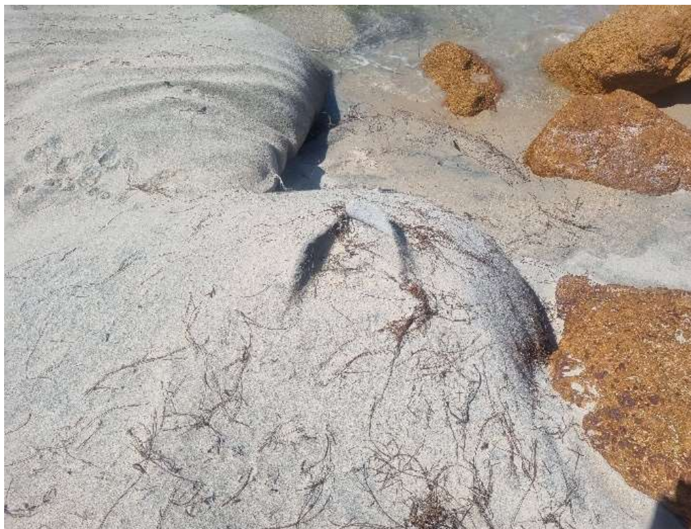
Figure 11-21: Ripped hole within GSC at Groyne 10 taken during site visit 27 November 2024.
