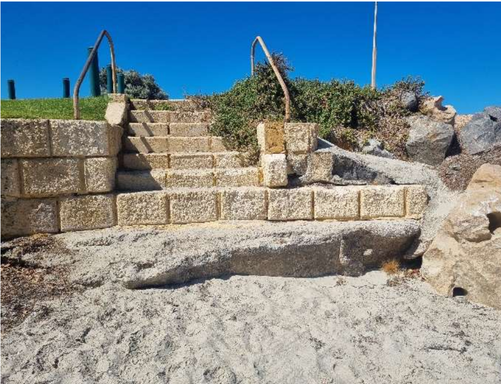
Figure 1-6: Ad hoc repairs of limestone stair access/retaining wall at Grannies beach (taken during site visit 29 January 2024)
