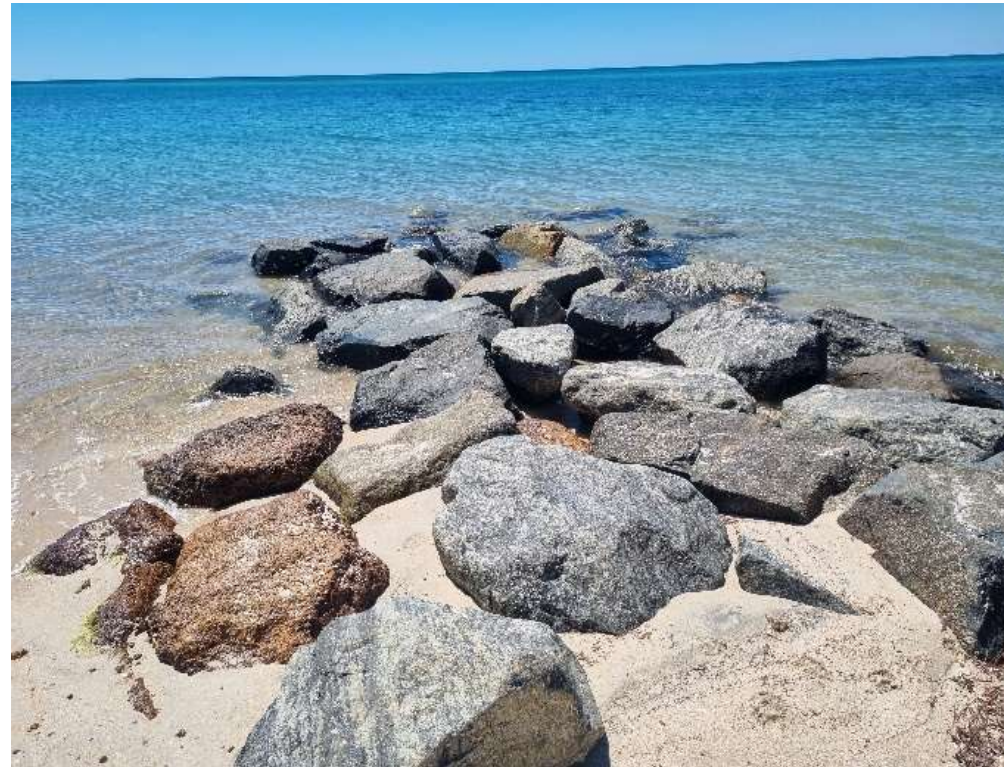
Figure 11-12: Groyne 4 taken during site visit 27 November 2024.
