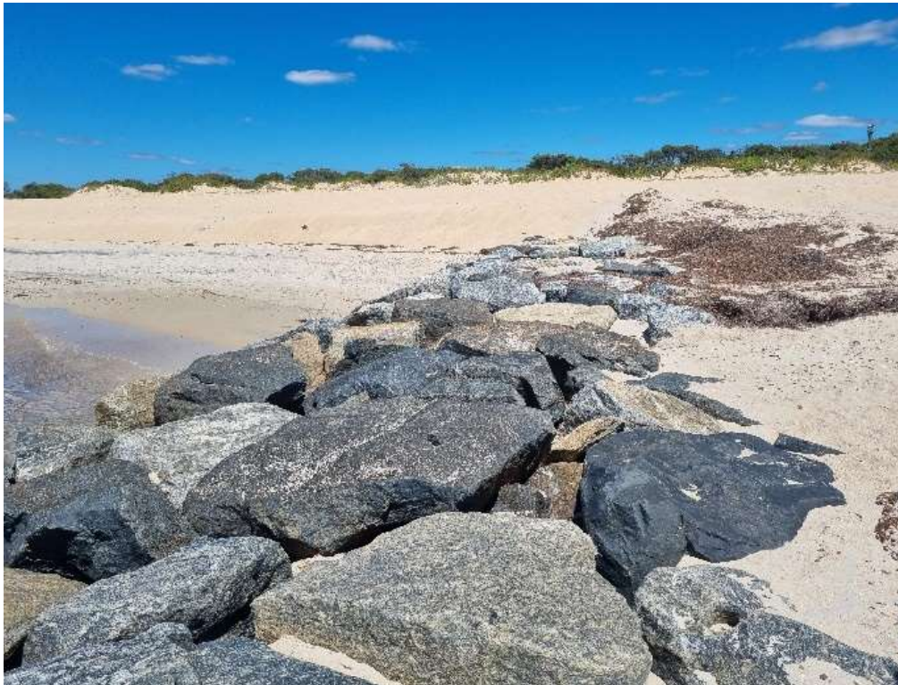
Figure 11-11: Groyne 4 taken during site visit 27 November 2024.
