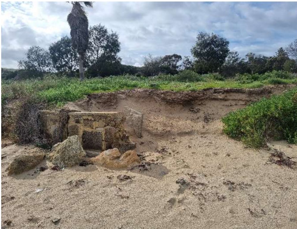
Figure 7-5: Photo taken of damaged limestone retaining wall (+1500m) with scattered armour loosely placed adjacent, facing east during site visit 14/08/2024.
