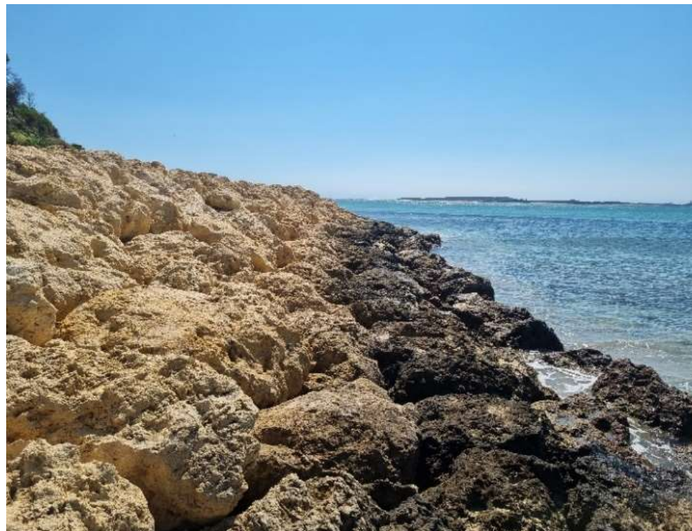
Figure 9-8: DBCA Revetment (+1150m). Taken during site visit 18 September 2024.
