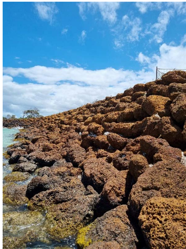
Figure 12-14: Seawall extending south-west of damaged section, taken during site visit 5 December 2024.
