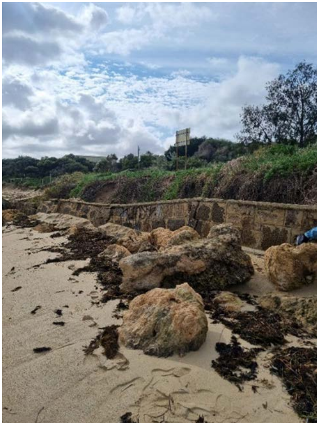
Figure 7-3: Photo taken of damaged limestone retaining wall (+1500m) with scattered armour loosely placed adjacent, facing east during site visit 14/08/2024.
