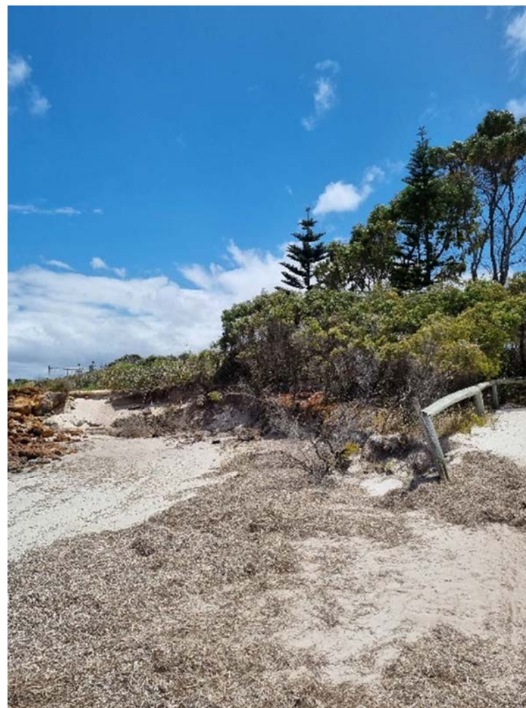
Figure 12-12: Damaged seawall and dune erosion (~+475m). Taken facing northwest during site visit 5 December 2024.
