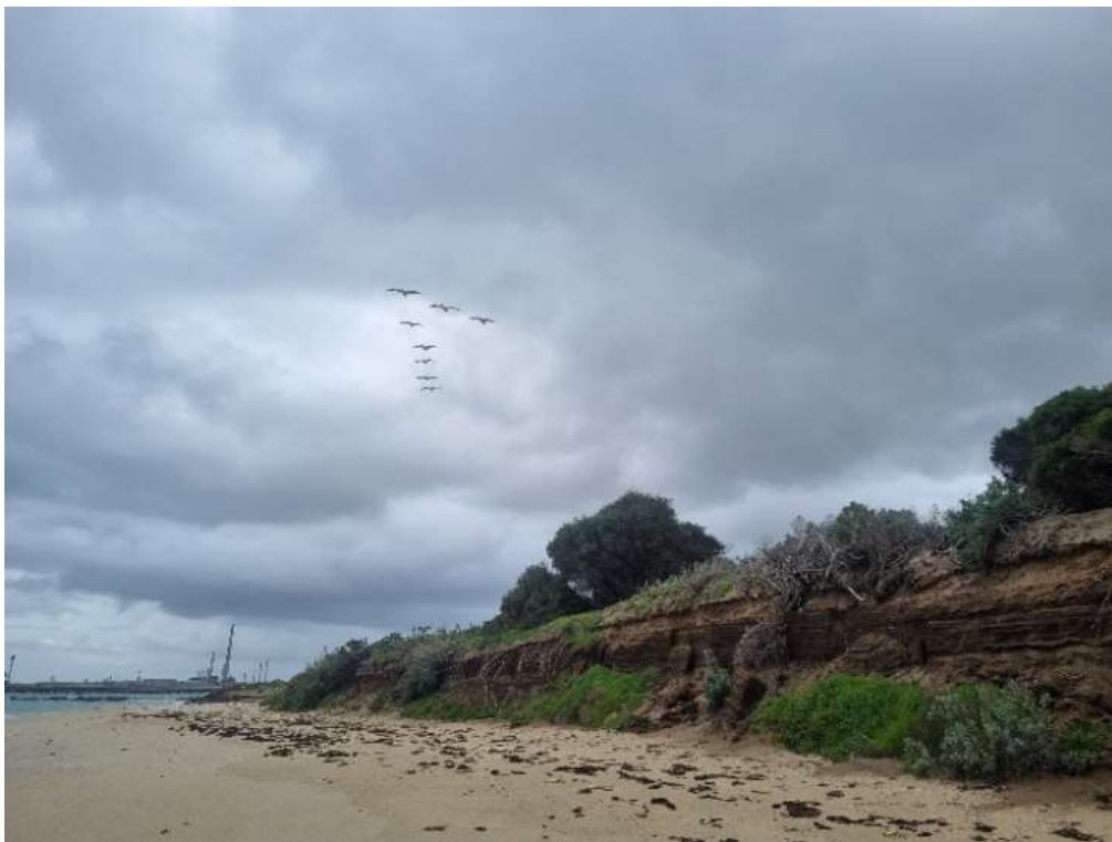
Figure 6-5: Coastal scarping and vegetation reestablishment along BP refinery foreshore (chainage +3000m), facing north during site visit 14 August 2024.
