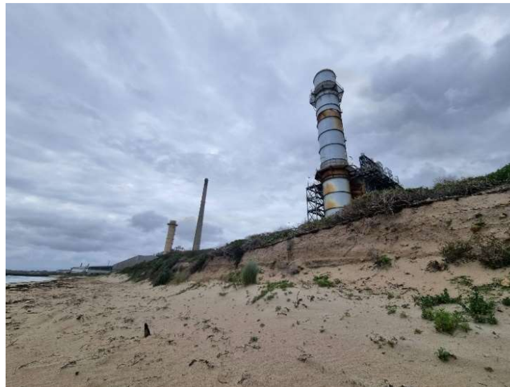
Figure 6-12: Scarping along dune face adjacent to NewGen power station (chainage +taken during site visit 14 August 2024.
