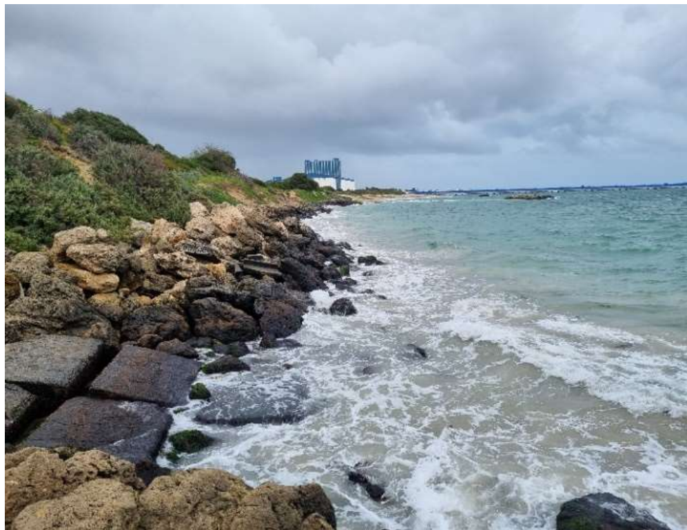
Figure 7-10: Limestone seawall south of Wells Park (+1100m), showing eroded dune face above, facing south during site visit 14/08/2024.
