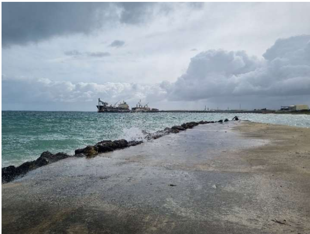
Figure 7-1: Photo taken of Wells Park headland (+1350m) showing overtopping during site visit 14/08/2024.
