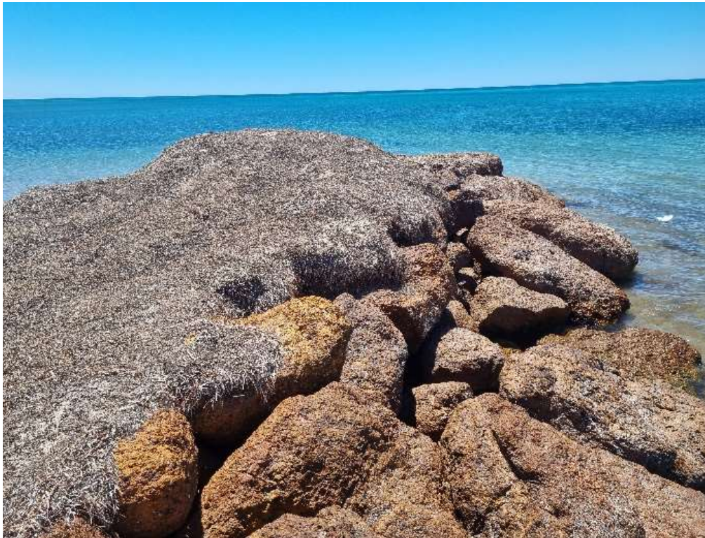
Figure 11-7: Wrack accumulated on crest of Groyne 2 (+350m) taken during site visit 27 November 2024.
