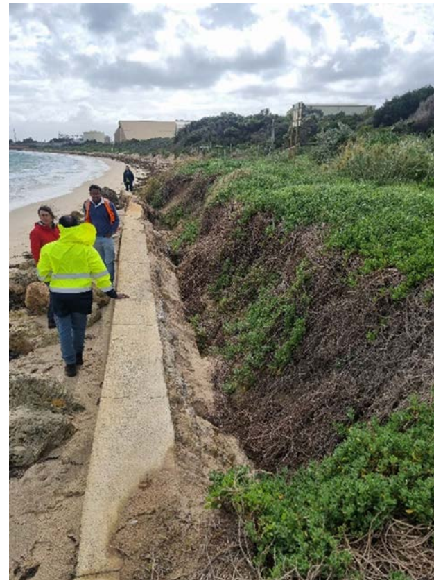
Figure 7-4: Photo taken of damaged limestone retaining wall (+1500m) eroded slope behind, facing northeast during site visit 14/08/2024.
