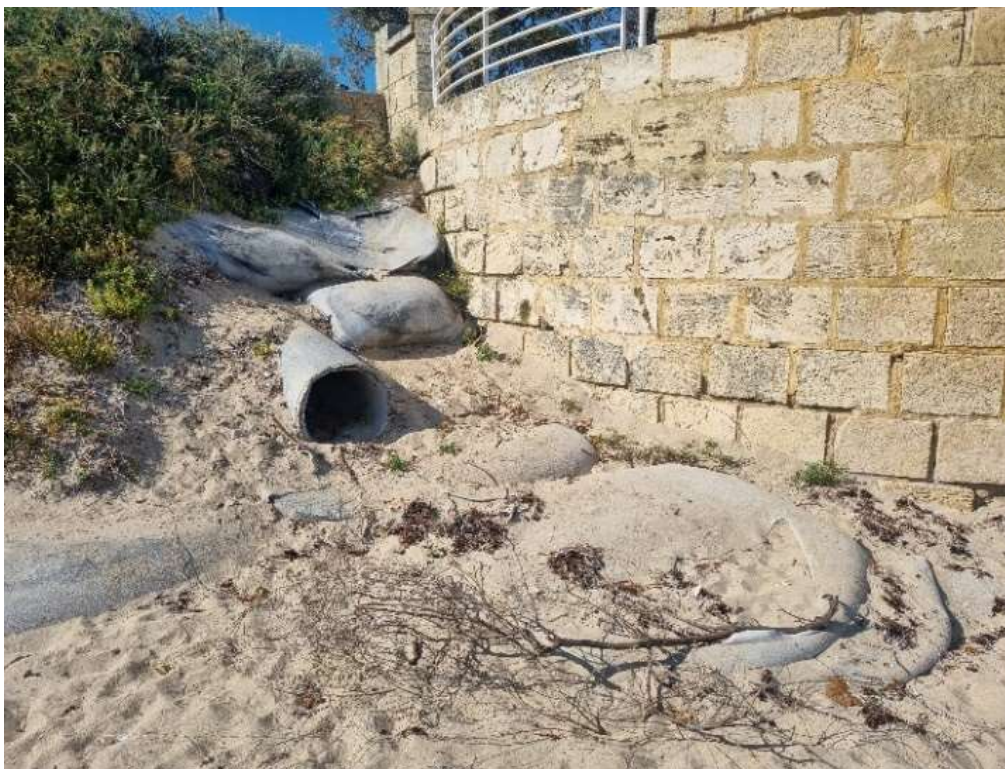
Figure 8-3: Photo taken of empty/damaged GSC within the Flinders Ln seawall, approximate chainage +3300 m. Taken during site visit 18 September 2024
