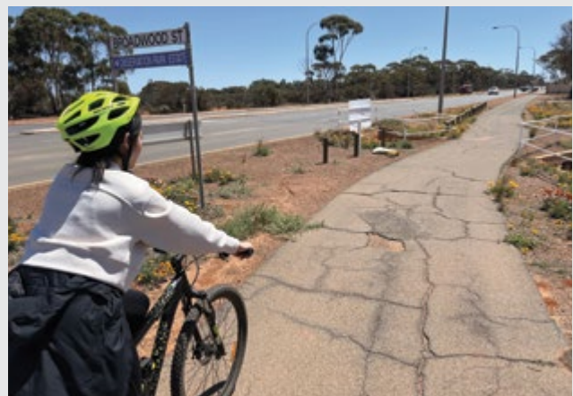
The shared path past Broadwood Street, which connects people to jobs in the West Kalgoorlie industrial precinct.
