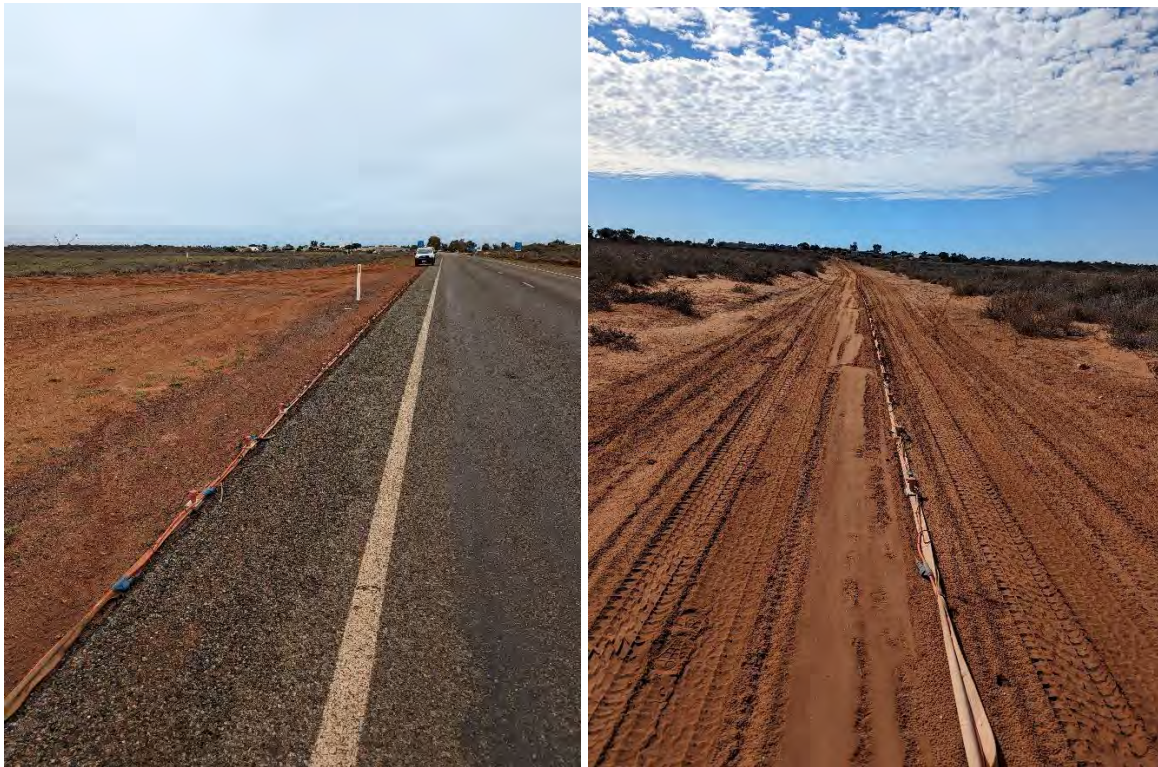
Figure 2: Site conditions at Onslow South along Onslow Road (left image) and unsealed foreshore road (right image).
