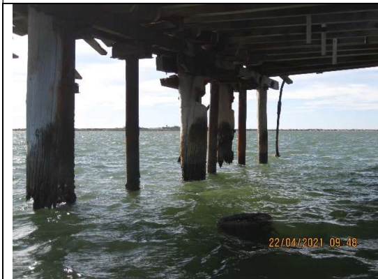
Photo 4: Underside of jetty head showing timber piles completely rotted at water line
