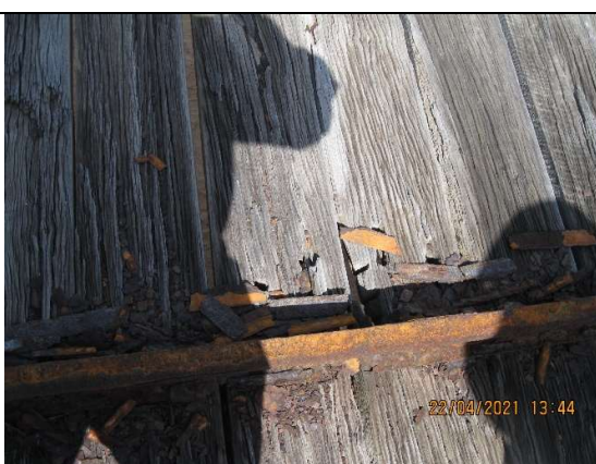
Photo 23: General deterioration of decking and rail line
