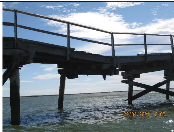
Photo 13: Missing pile and cross braces
