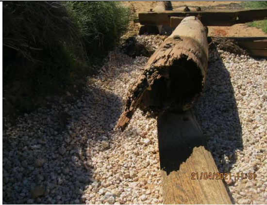
Photo 31: Salvaged timber piles still attached to broken crossheads. Pile at top of photo has rotated. Both piles snapped at mid tide level due to rot and attack by marine organisms - predominantly Limnoria.
