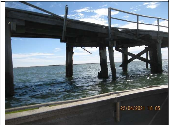
Photo 12: Broken Stringer and missing braces
