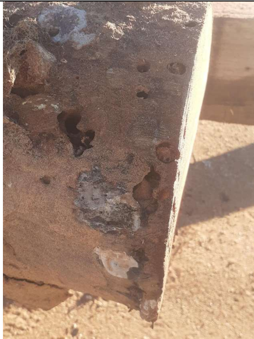
Photo 33: Same Pile with rotted section cut off to determine extent of Teredo Infestation.
