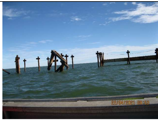
Photo 5: Broken Pier showing broken timber pile with crosshead still attached to steel pile
