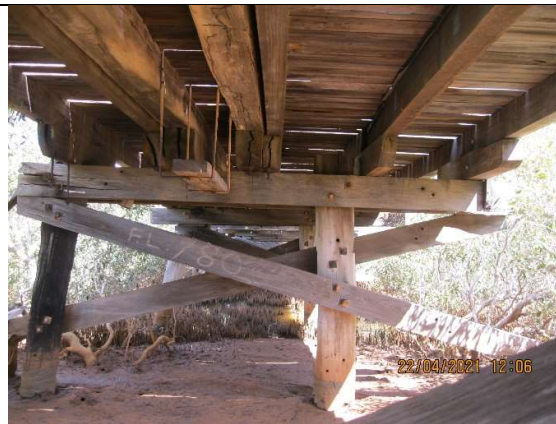
Photo 19: Abutment pile showing evidence of previous fire. Note also split corbel which is prevalent throughout.
