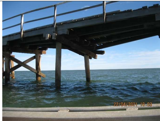
Photo 11: Broken pile causing jetty to collapse
