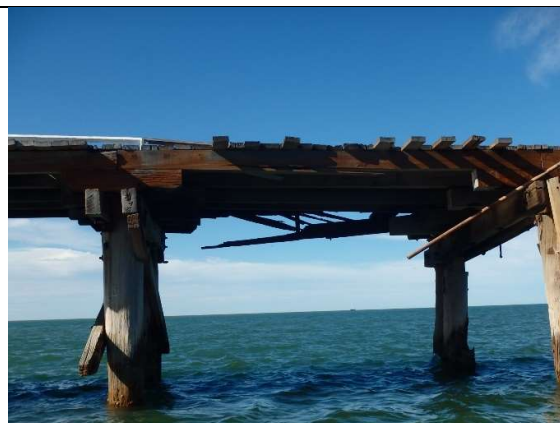
Photo 15: Broken Stringer and missing handrail
