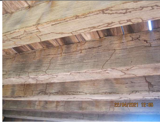
Photo 17: Evidence of termite on stringers near abutment
