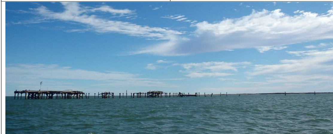
Photo 3: Panoramic view of jetty head and end of approach jetty showing missing sections
