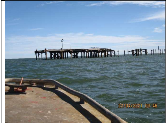
Photo 1 Jetty Head - 5 bays remaining.
