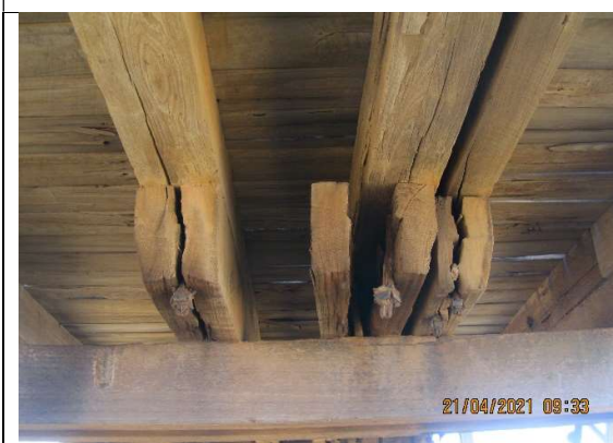
Photo 24: Typical detail of split corbels resulting in separation of corbels and stringers from the crossheads
