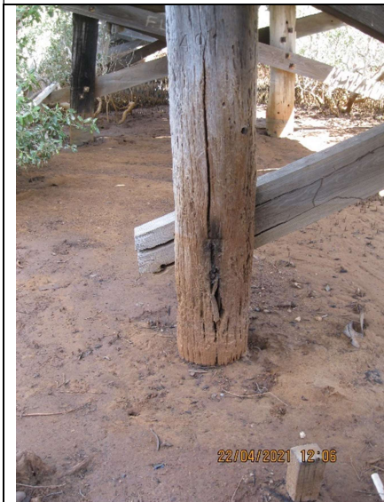
Photo 18; Pile near abutment showing evidence of rot. Likelihood of necking below the mudline when mud level was lower.
